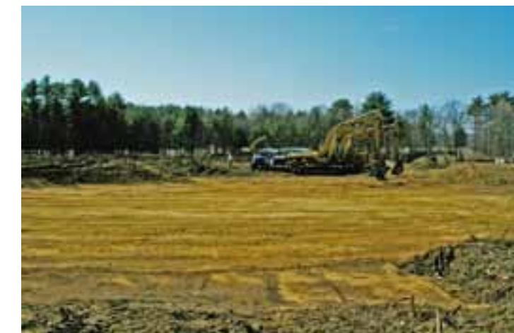
Initial site work for the new Keene Middle School is nearly complete. It has transformed that section of Maple Avenue.
